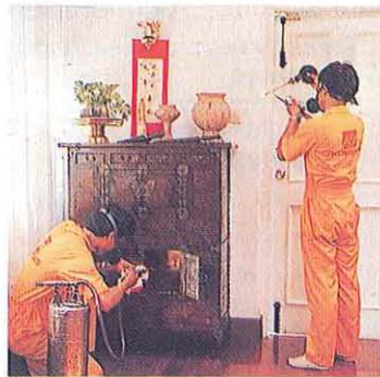
Termite control in the house
