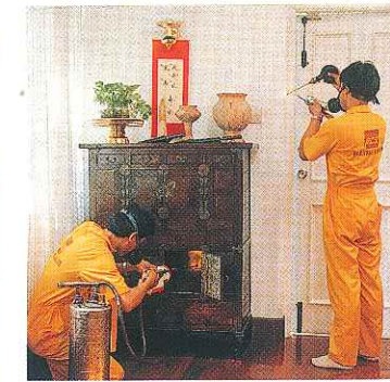
Termite control in the house
